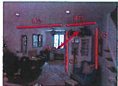
Picture 6: Partition wall to be removed PW-2 around kitchen (view from family room)
