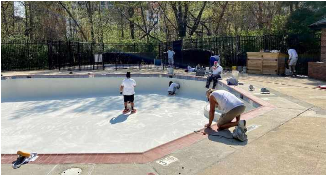
In the photo above on April 6, Wilcoxon, whitecoat/plaster subcontractor for Premier Aquatics applies a new whitecoat to Pool 6. Whitecoats typically last 5-7 years depending on conditions and are included in our reserve study. Whitecoating is a reserve expense.
