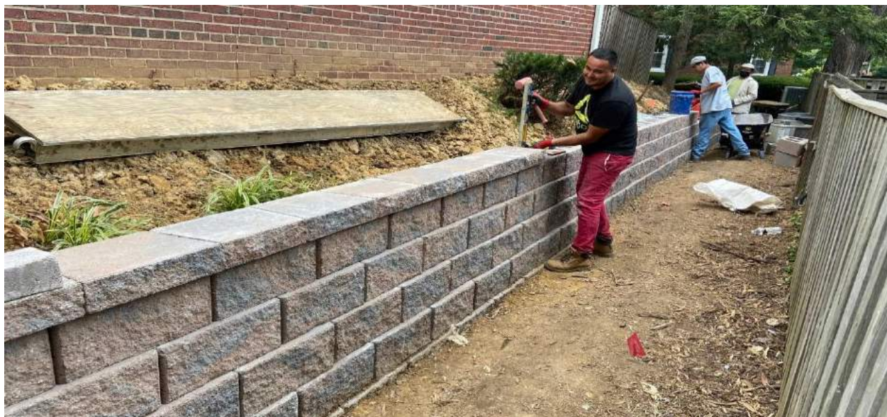
In the above photo, American Restoration nears completion on the 31 st Street retaining wall.
