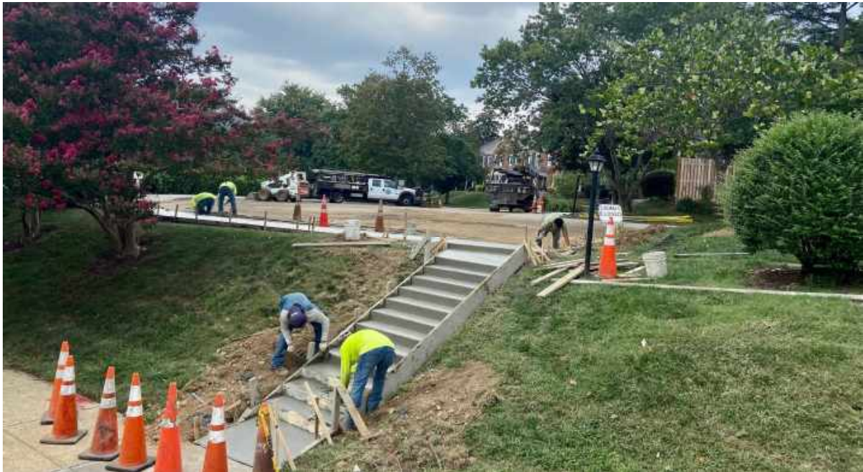
In the above photo, Edge Concrete replaces the steps and perimeter sidewalks in parking lot 53 (4652-4654 S. Abingdon Street). Drainage is also greatly improved now in this lot after the change of several elevations.
