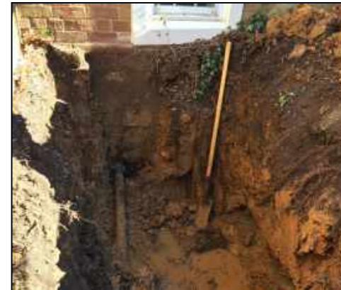
Water Lateral Leak
