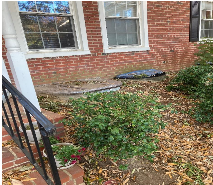
Figure 1 Egress window next to standard window
