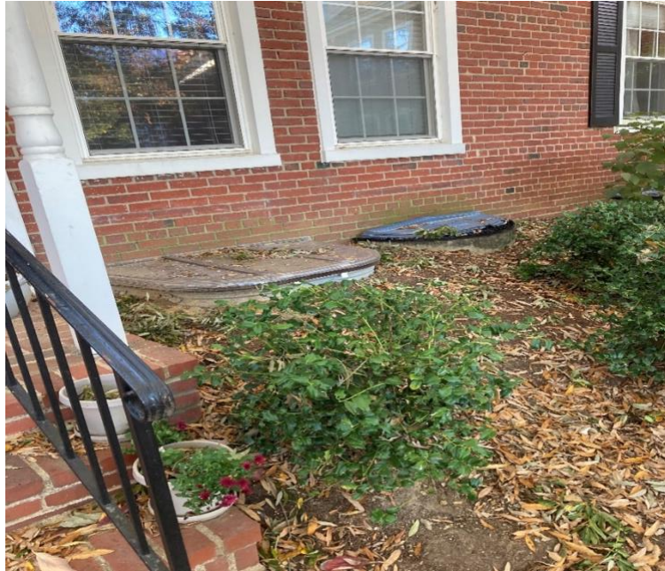
Figure 1 Egress window next to standard window
