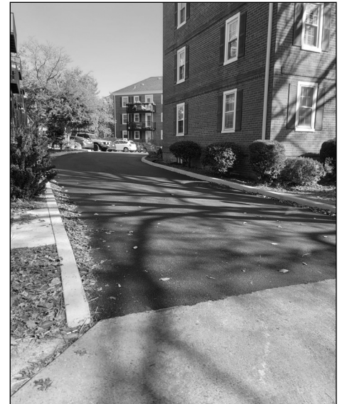
PHOTOS BY MANAGEMENT At left: a new sidewalk; above: a parking lot renovation.
