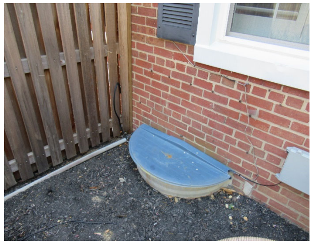
Photograph #4: Window well with plastic cover
