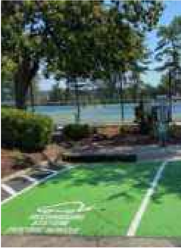
Two electric vehicle chargers located in the Community Center parking lot can be used by residents for a nominal fee. Photo by Mark Johnson.
